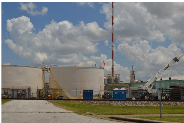
Storage tanks proved to be one of the most vulnerable pieces of industrial infrastructure during Hurricane Harvey, with more than two dozen tanks leaking toxins into the air and water.
