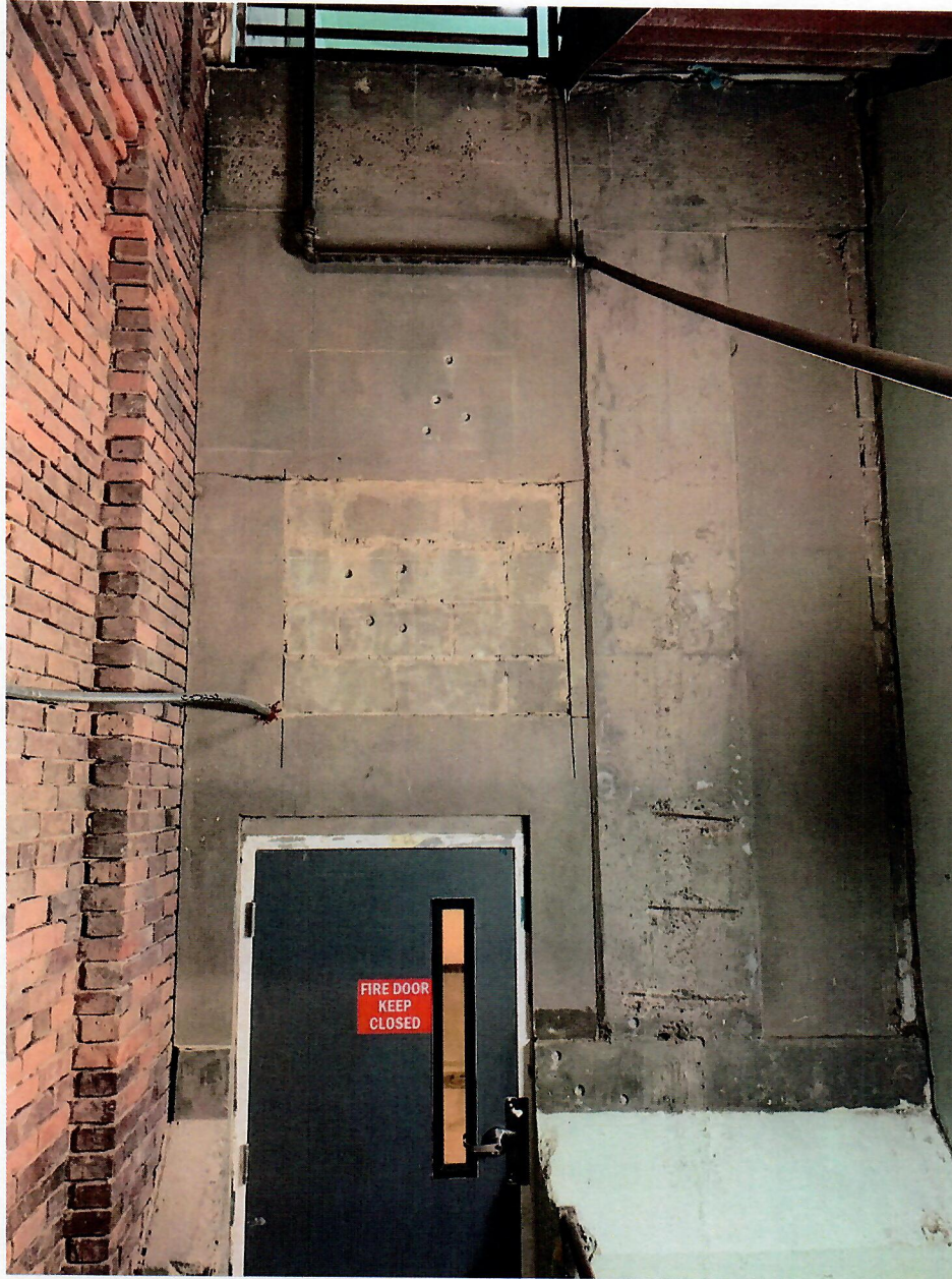
BUILDING 22, 6 TH FLOOR, WEST ELEVATION. CLOSE-UP OF CONCRETE WALL INCLUDED IN SET-UP #39.
