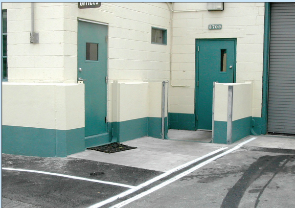
Figure 3-12. Front of retrofit dry floodproofed building where drop-in flood shields protect doors
