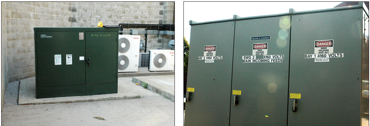
Figure 4-19. Pad-mounted transformer (left) and 15 kilovolt switchgear (right), both vulnerable to damage when inundated with floodwaters (Cedar Rapids, IA, 2008)
