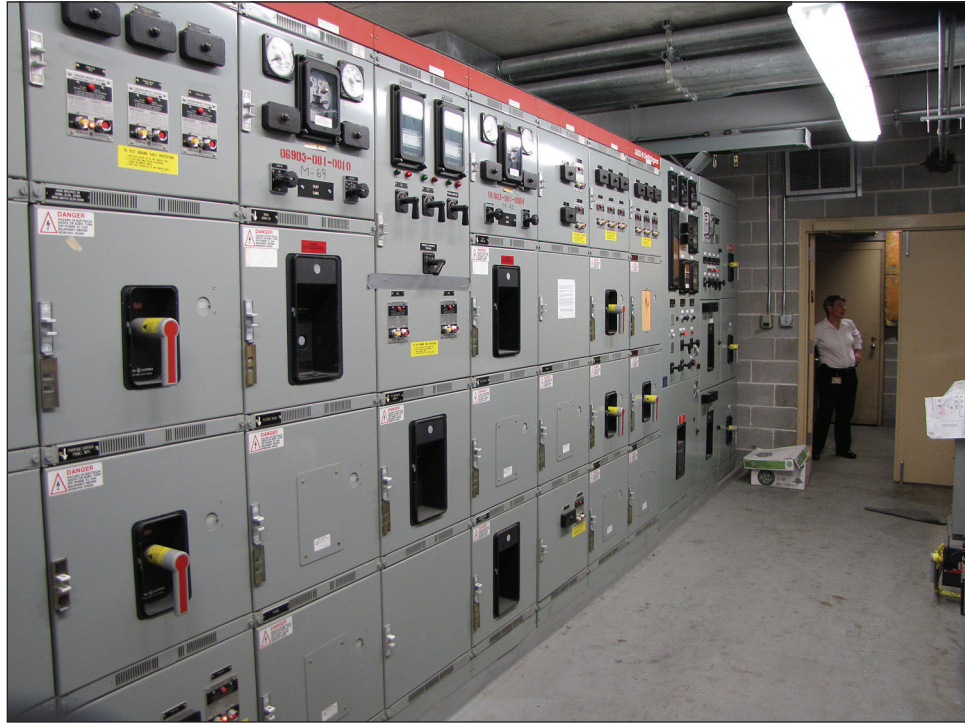
Figure 4-17. Undamaged secondary switchgear located at the University of Texas Medical Branch. The switchgear had been constructed on an upper floor that remained above flood levels. The switchgear was not damaged during Hurricane Ike (Galveston, TX, 2008).
