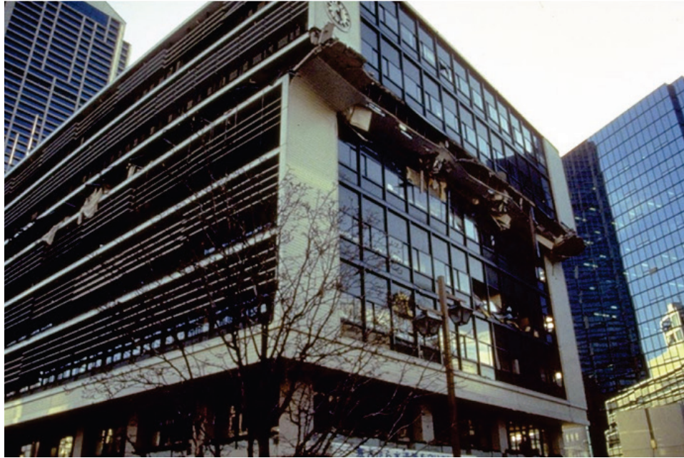
Figure 3-15 Sixth story collapse of 8-story Kobe City Hall Annex building in 1995 Kobe Earthquake in Japan (Source: EERI Slides on the Hyogo-Ken Nanbu (Kobe) Earthquake of January 17, 1995).
