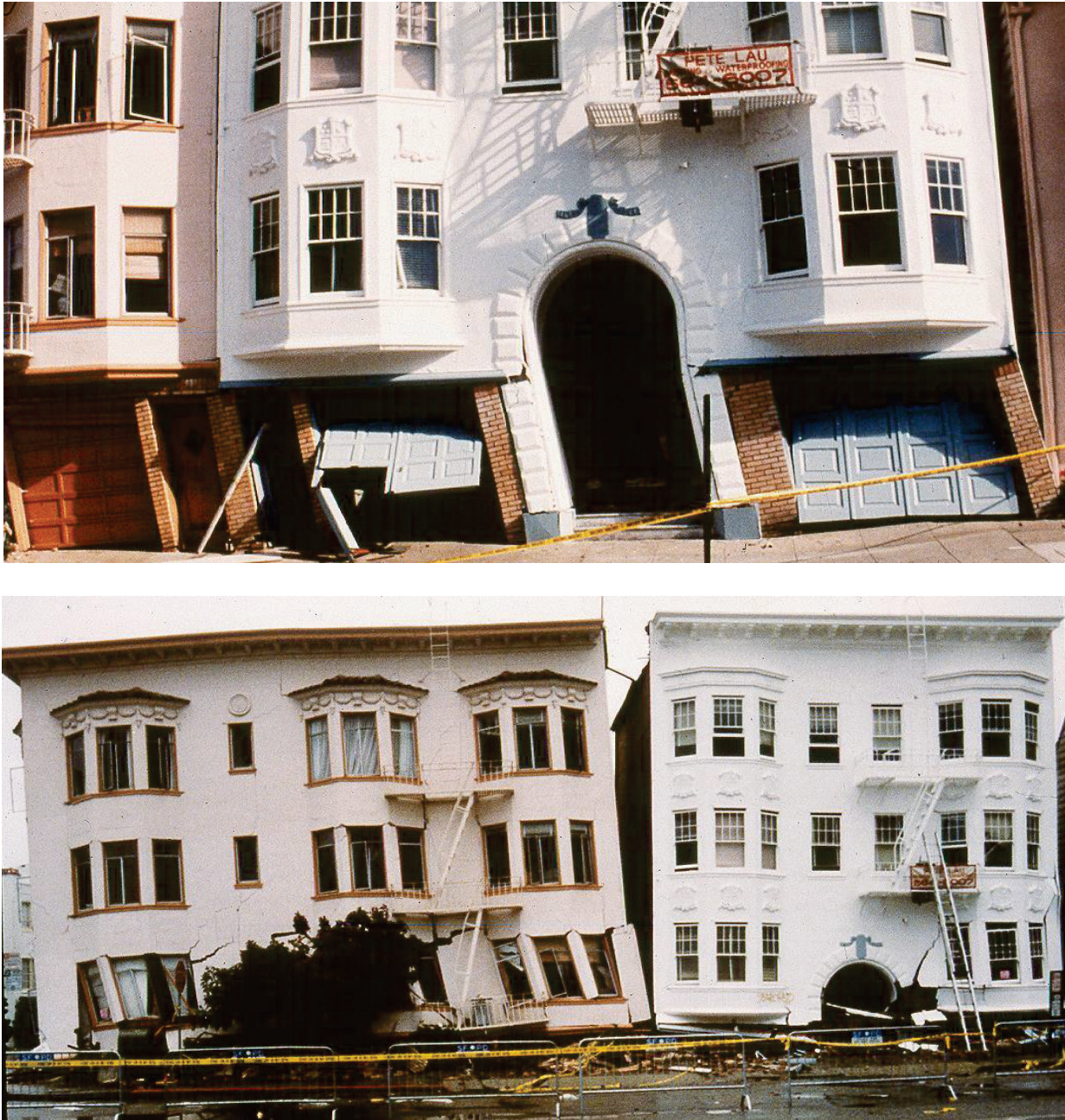
Figure 3-13 San Francisco soft story collapse showing leaning story after main shock (upper photo) and story collapse in aftershock (lower photo). Image from ATC-20 training materials.
