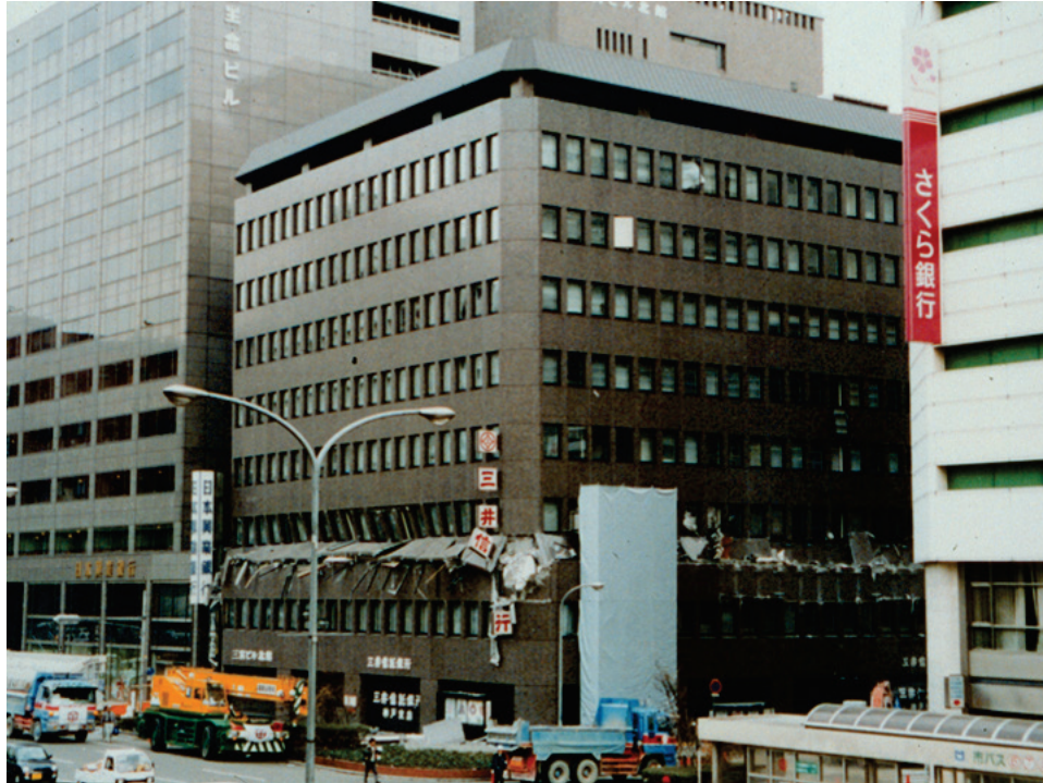
Figure 3-14 Third story collapse of 10-story office building in 1995 Kobe Earthquake in Japan (Source: Exponent/Osteraas).
