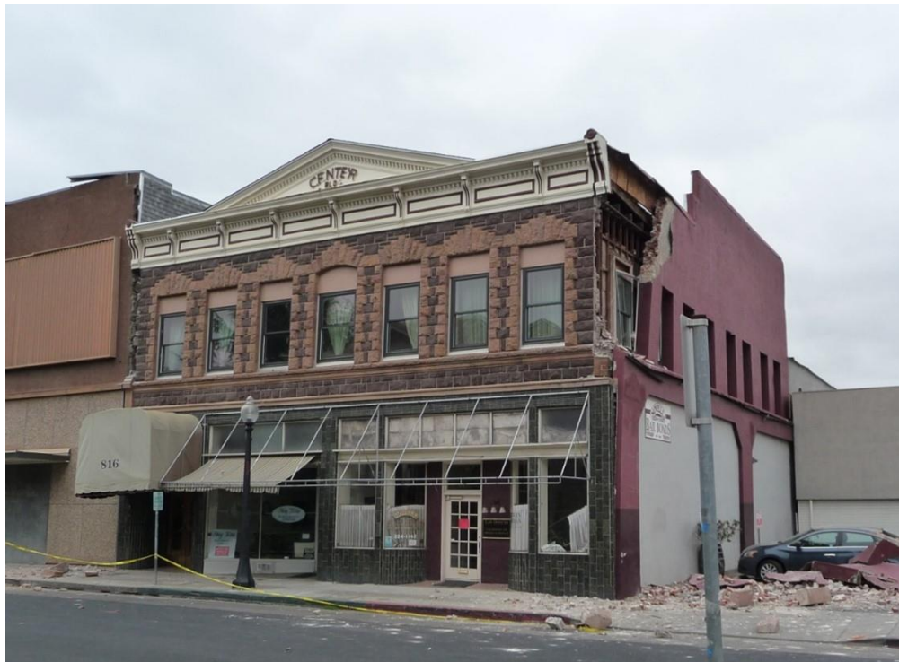
Figure 2-4 Failure of URM south wall of URM building posted UNSAFE (FEMA P-1024 Figure 4-49, photo by Marko Schotanus).
