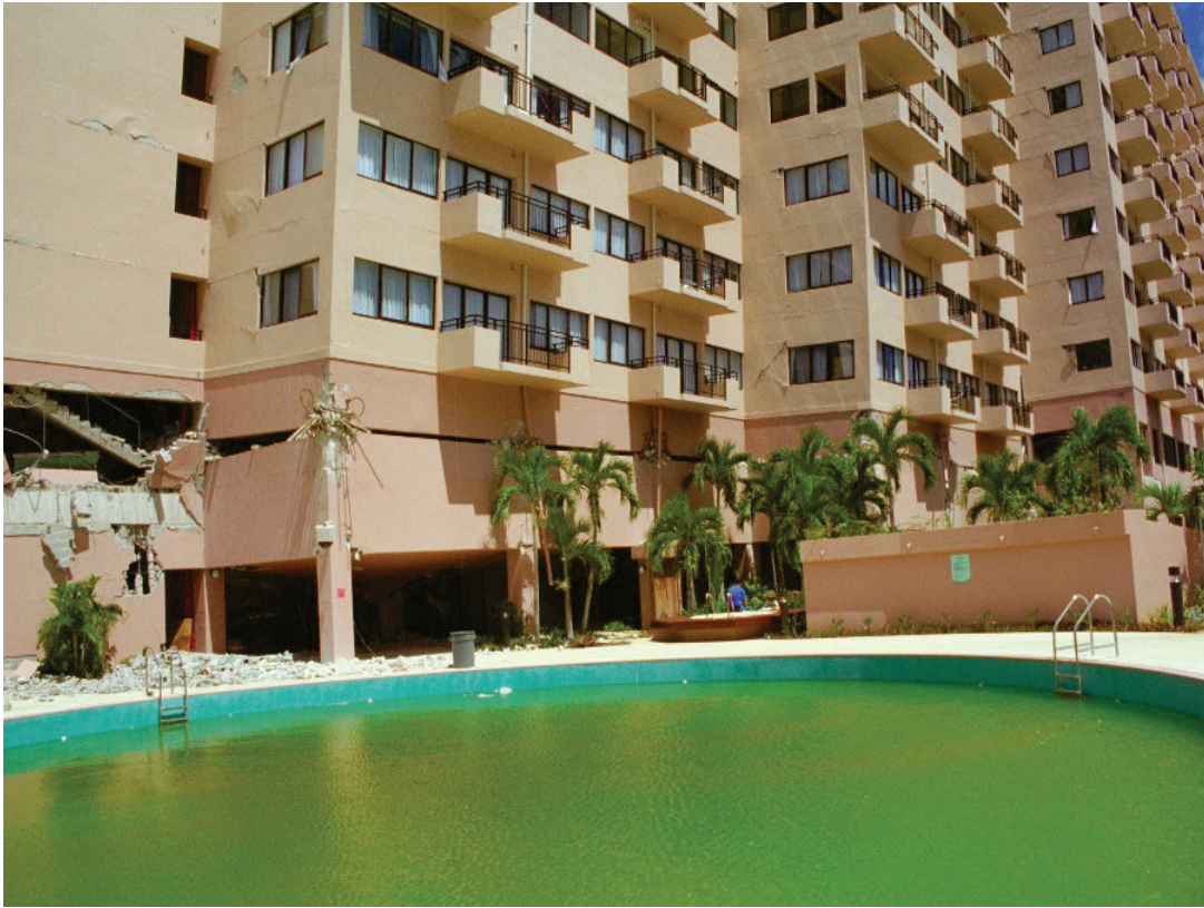
Figure 3-7 Partial collapse of Royal Palm Resort in 1993 Guam Earthquake due to shear failure of captive columns in soft story. Note undamaged adjacent structure along right edge of photo (Exponent/Luth).
