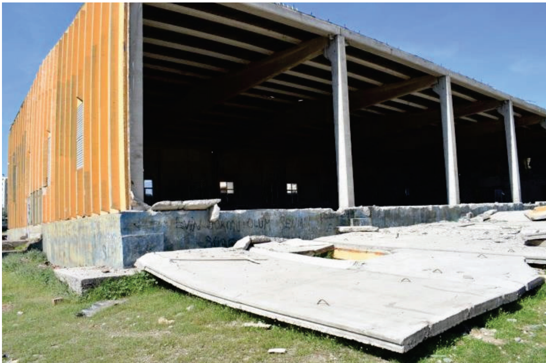
Figure 3-30 Warehouse in Kahramanmaraş after the 2023 Kahramanmaraş Earthquake (Türkiye). (Photo Credit: Thornton Tomasetti/Galvis).
