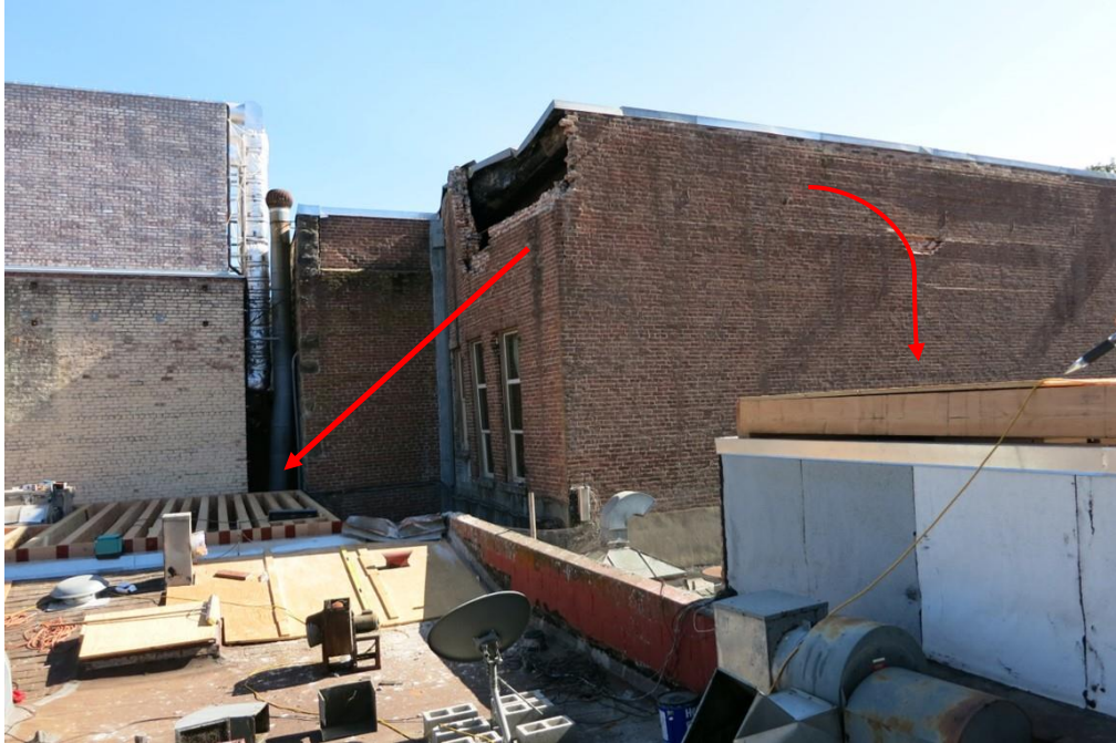
Figure 2-5 Protective barrier constructed over the rooftops of buildings to protect from falling brick. (FEMA P-1024, Figure 12-7)
