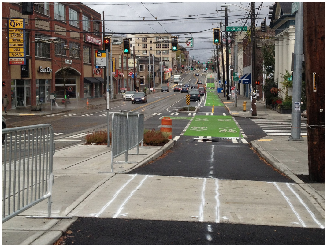
Raised crosswalk (under construction) adjacent to a transit stop island platform on Broadway in Seattle, WA. (Source: Seattle DOT)
