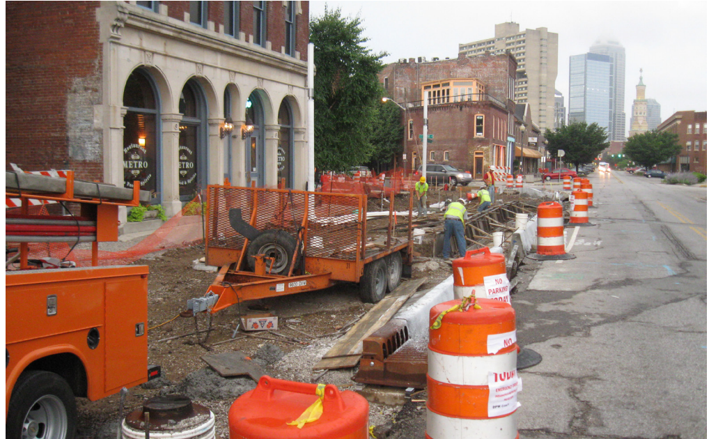
Construction of the downtown Cultural Trail in Indianapolis, IN. (Source: Mark H. Zwoyer)
