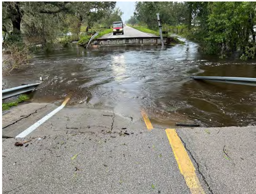
Figure 36. Hollandtown Road in Hardee County washed out by Hurricane Ian
