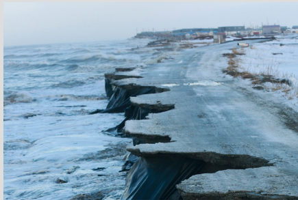
Damage to Shishmaref sanitation road
