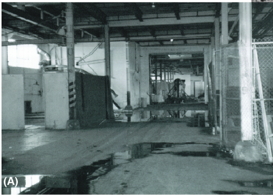
(A) The interior of one of the piers at Fort Mason prior to renovation.
