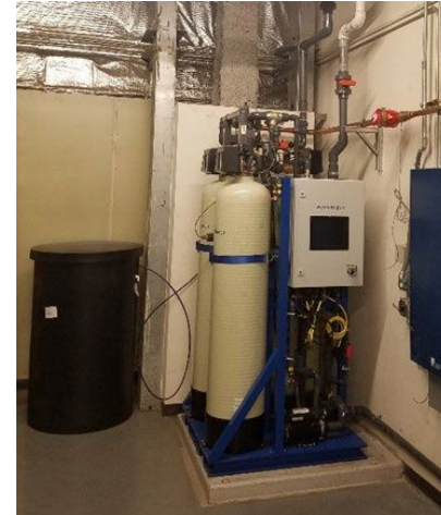
PWS system Lloyd D. George U.S. Courthouse
