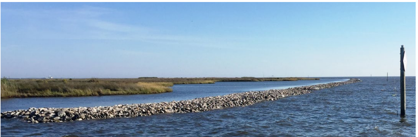
The Hancock County Marsh Preserve in Hancock County, Mississippi where 6 linear miles of living shoreline were built between 2017 and 2018. The living shoreline protects coastal marsh habitat from erosion and also serves as habitat for oysters and other benthic fauna ( DIVER ID 38 ).
