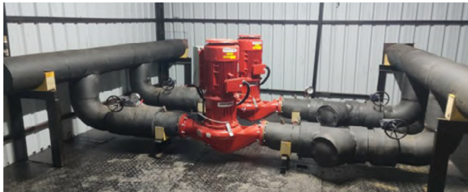
Armstrong Pumps: Chilled water pump and condenser water in India
