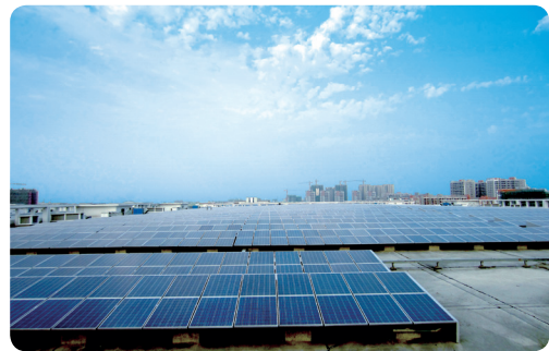
Solar power stations at Huawei's Dongguan Campus
