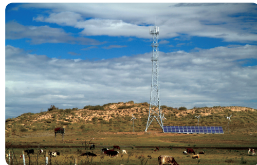
Solar-powered base stations in Inner Mongolia, China
