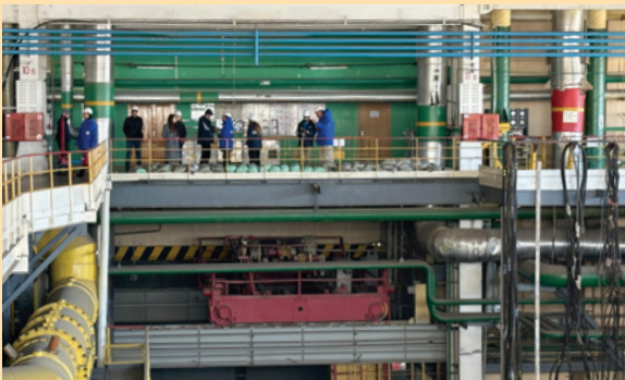
IAEA team conducts a walkdown in the turbine hall of Unit 4 (Photo: IAEA)
