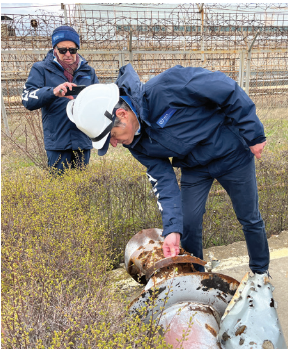
29 March 2023: The second visit was to witness the damage to the ZNPP that had occurred since September 2022, in particular that associated with the reported shelling in November 2022 (Photo: IAEA)
