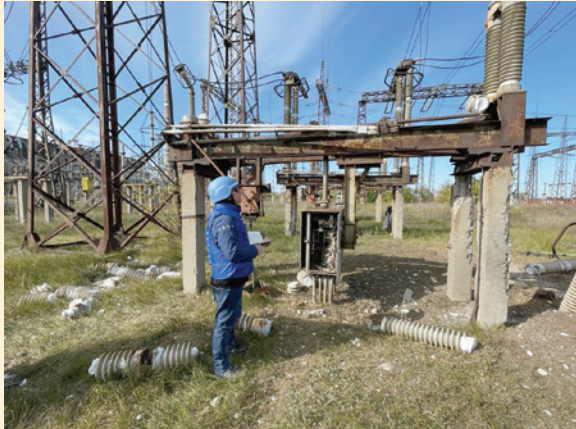
IAEA team conducts a walkdown of the ZTPP 330 kV switchyard after damage by reported shelling (Photo: ZNPP)
