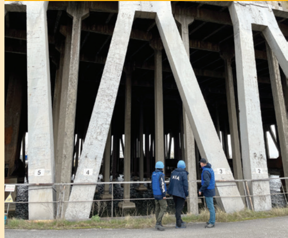
IAEA team conducts a walkdown of the cooling towers at the facility (Photo: ZNPP)
