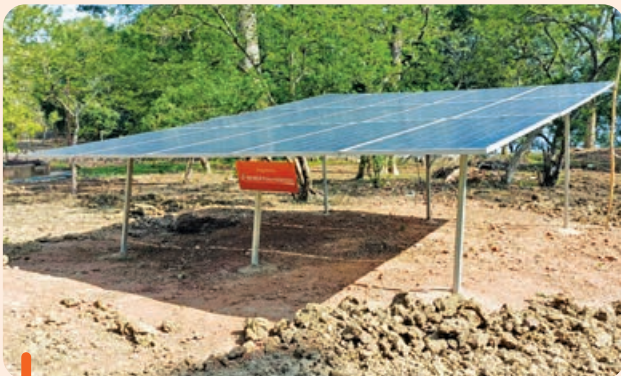
A solar panel installed at Tadoba-Andhari Reserve, Maharashtra
