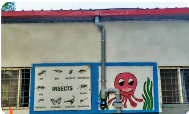
Rainwater harvesting pipes installed at an Army Public School in Pune, Maharashtra
