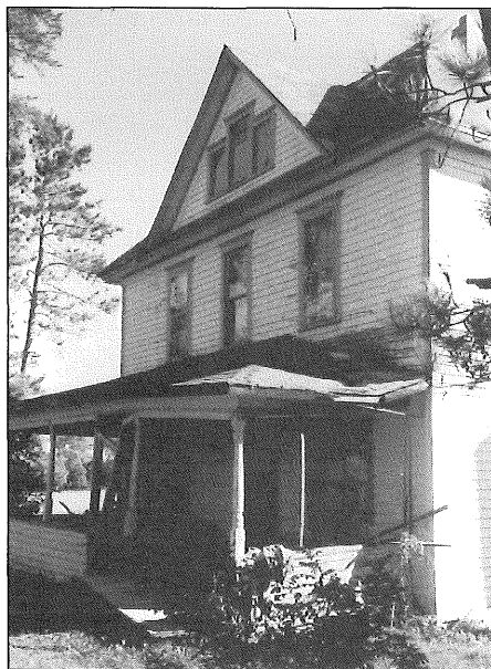
The elderly woman who owns this home will have to wait until 2001 to get her leaky roof replaced. Pat Alberg distributed this photograph to members of the Housing Committee at the Park Rapids hearing stressing that government needs to be more flexible in looking at the problems of individuals.
