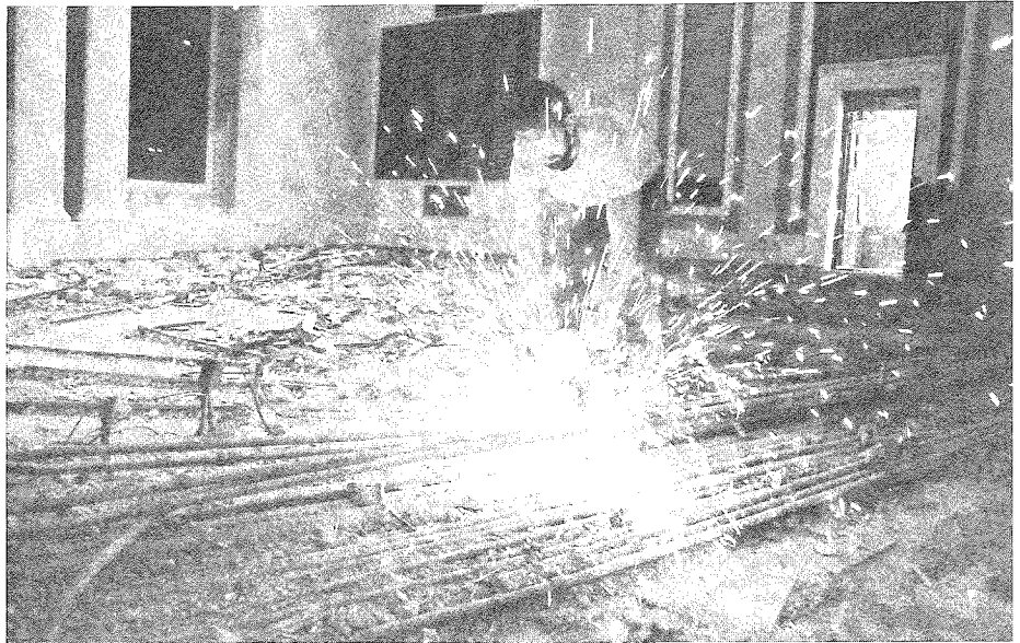
Sparks flew in the House Chamber Aug. 22, but not because of a proposed tax plan. Jerry Rock, an employee of Peoples Electric Co., cut electrical conduit during demolition of the Chamber. Workers are remodeling the House Chamber during the interim. Target date for completion is Feb. 12, 1990, when the House reconvenes for the second half of the regular legislative session.
