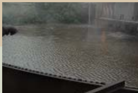
The thickener (above) separates the process water from the concentrate, allowing the water to be reused.
