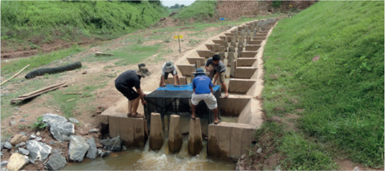
Vertical slot fishway structure constructed in May 2019 at the Kbal Hong Weir in Pursat Province, Cambodia.
