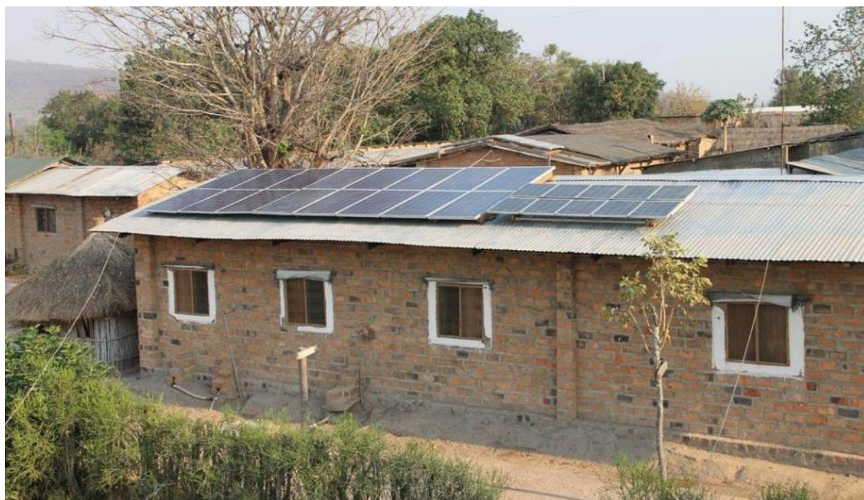
An MSF team installing solar panels on the roof of Shamwana health centre to make sure electricity remains on in the hospital and keeps the cold chain running. This will replace approximately 1,000 litres of diesel per month. Photo: Per-Erik Eriksson/MSF.
