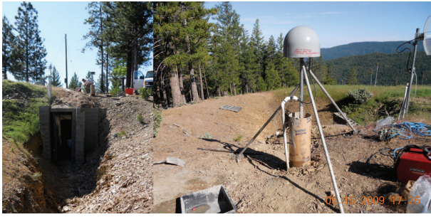
Figure 3.24: Site GASB in Alder Springs, CA. Left: Wide view showing seismic vault, which is cemented to bedrock. Right: Close-up of monument during pouring of stabilizing cement; the central support mast was embedded in the wall of the seismic vault during construction.
