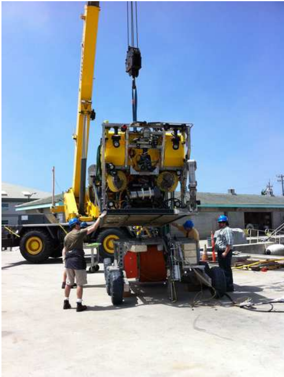
Figure 3.7: This figure shows the cable laying tool, with the red cable wrapped inside it, as it is being mounted on the bottom of the ROV Ventana prior to installation. The sharp metal "edge" hanging from the middle of the sled was used to dig a narrow trench in the seafloor as the cable was laid down, so as to bury it and protect it from trawling,. Courtesy of Paul McGill, MBARI.
