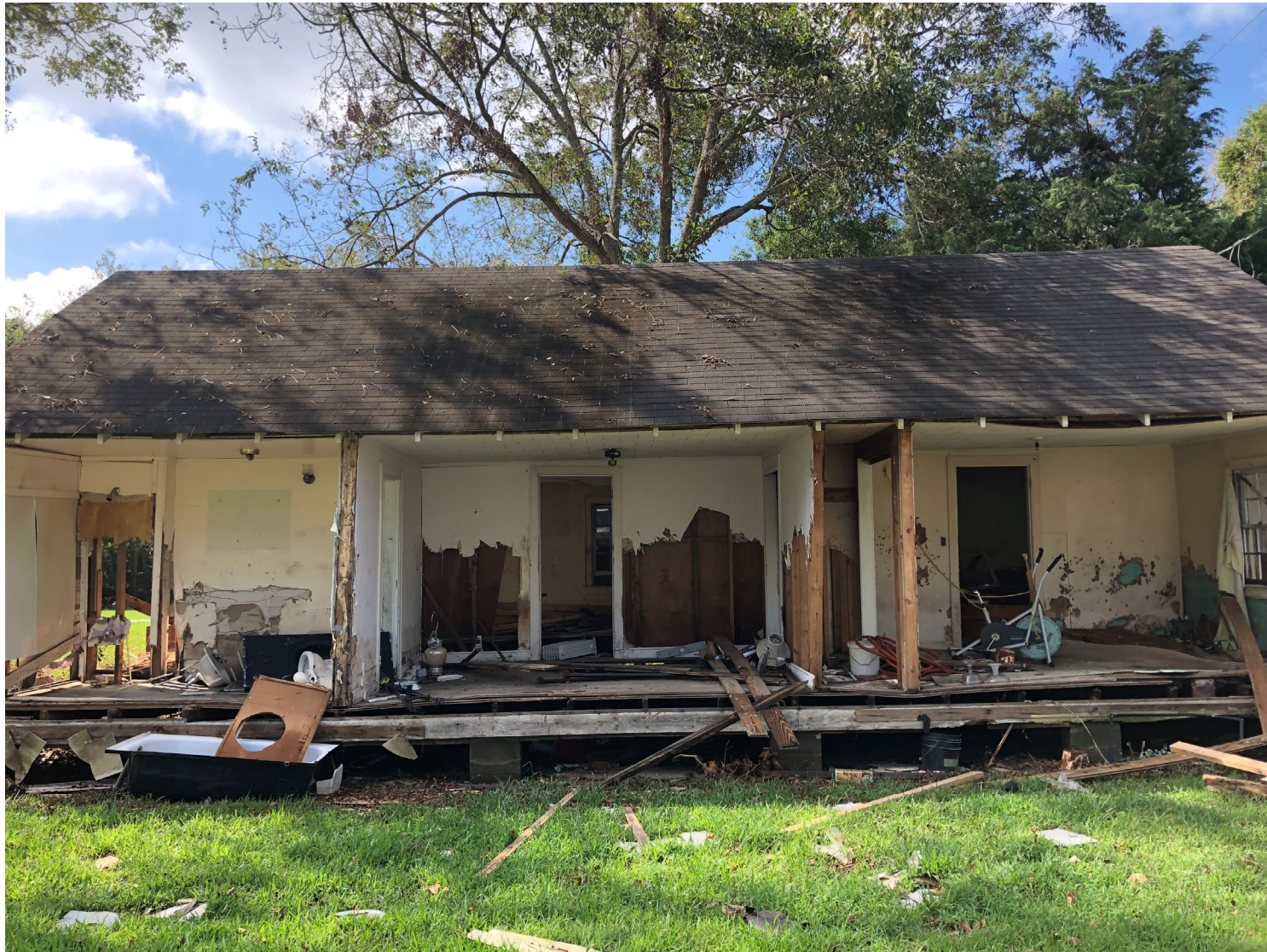
Figure 14. House severely damaged by storm surge in New Bern, North Carolina.
