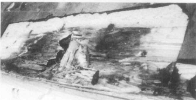
Figure 15. (a) A regular cleaning schedule would have eliminated the plant growth and leaf build-up in this gutter, which, if not removed, will result in serious damage to roof sheathing and structure (b). Photos: (a) Paul K. Williams, and (b) Walter S. Marder. AIA.
