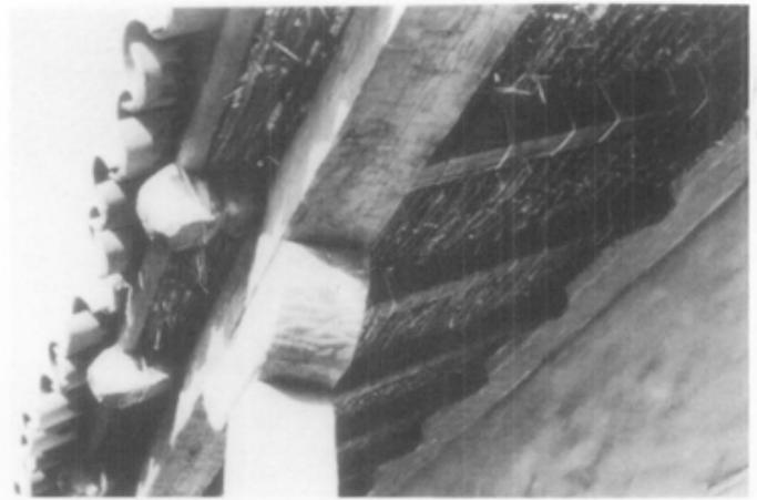
Fig. 10. The underside of this roof on the restored barracks at Santa Cruz Mission reveals the twig sheathing or latia to which the clay tiles were traditionally attached with mud mortar. Photo: Gil Sánchez, FAIA.
