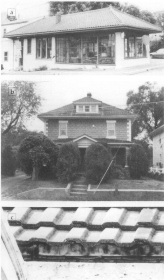
Fig. 7. (a) Metal "tile" roofs of galvanized steel closely resemble the clay tiles they mimic. Often painted to look like terra cotta, their identity can sometimes be revealed by peeling paint or dented "tiles." (b-c) Concrete roofing tiles are generally thicker than clay tiles, and tend to fade and lose their color. Photos: (a-b) Anne Grimmer, (c) National Park Service Files.
