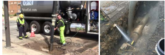
Figure 5: Using a hydrovac truck for inspection, requires a large truck and crew (left) and exposes the pipe material underground (right).
