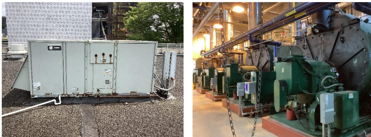
Figure 32 Typical Packaged Roof Top Unit ( left ) and Steam Boiler ( right )
