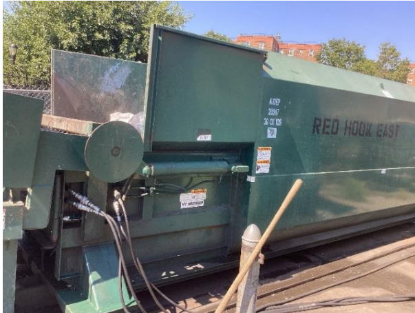
Figure 41 Typical Exterior Compactor
