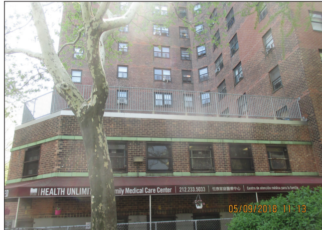
Figure F11. Lower roof area at LaGuardia Houses
