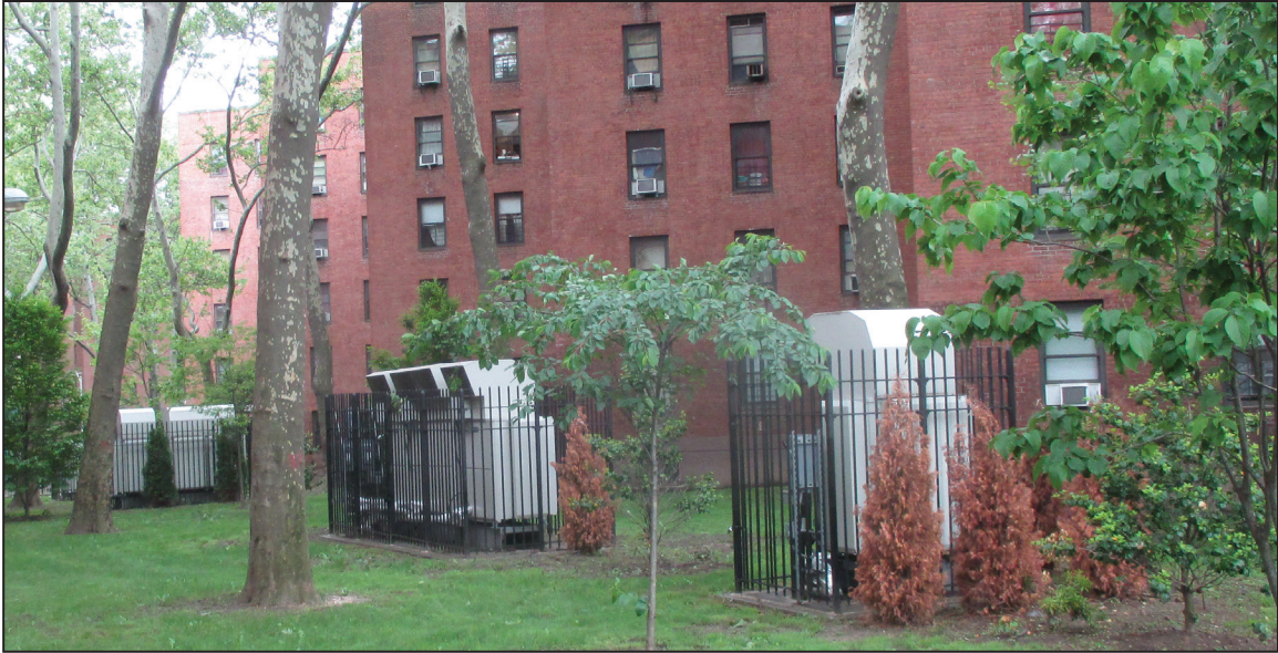
Figure F8. Heat pump outdoor units on the lawn at Vladeck Houses serving non-residential community spaces
