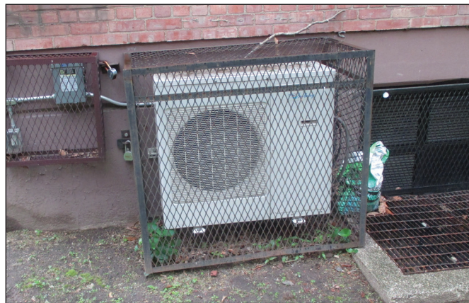
Figure F10. Heat pump outdoor unit mounted to the building exterior at Vladeck Houses
