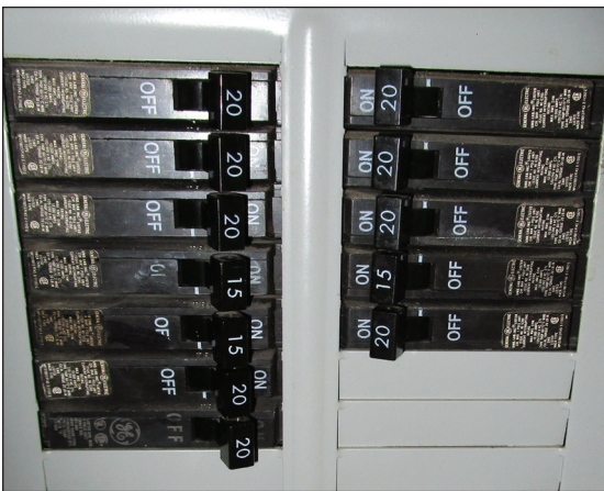
Figure A2. Some apartment panels, like this one, will have space for new breakers; others will not (Photo: Sahagian)
