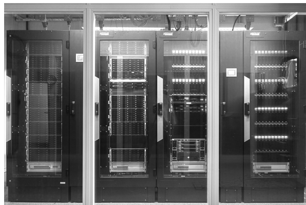
Fig. 1 Photo of the MPIfR HPC cluster. The 2 racks on the right house the compute nodes, head nodes, and network switches. In the 2 racks on the left are the RAID systems.
