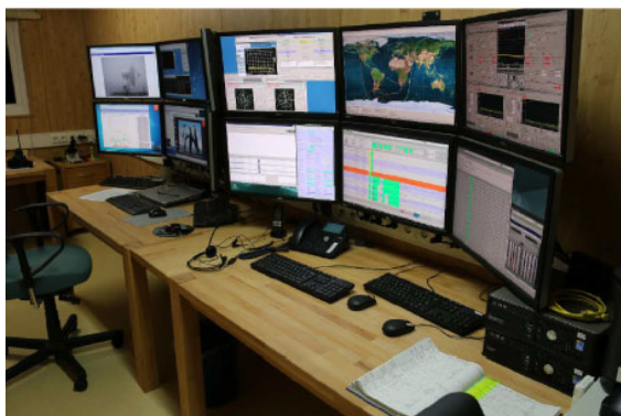
Fig. 4 New combined satellite tracking and VLBI control room.
