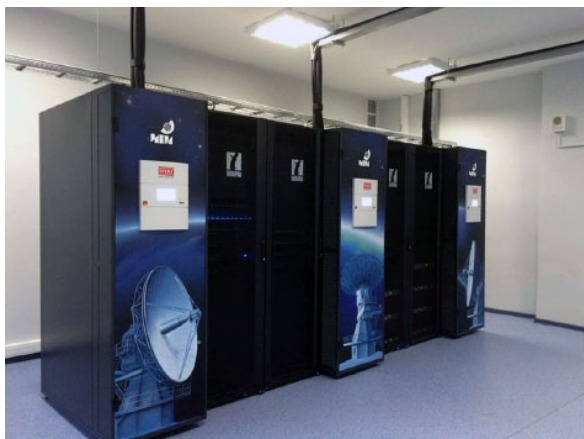
Fig. 7 High-performance computing cluster in St. Petersburg.
