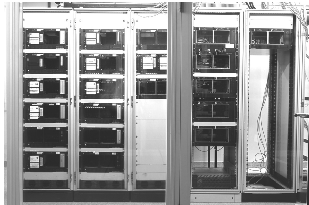
Fig. 2 Photo of the new chamber for the Mark5 and Mark6 units. The first Mark 6s are in the two racks on the left.
