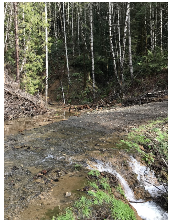
Road Washout of the 100 Rd
