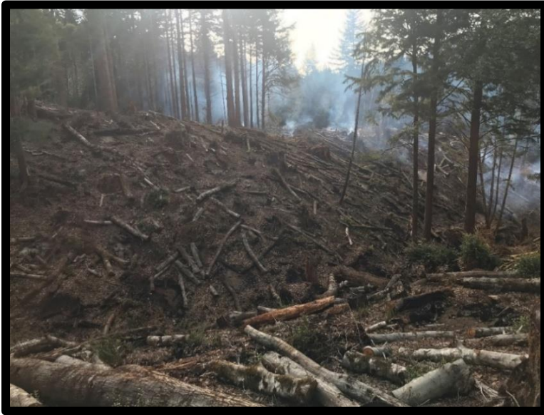
Treatment Unit at Humbug
