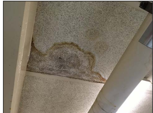
Water Damage at Roof Deck
