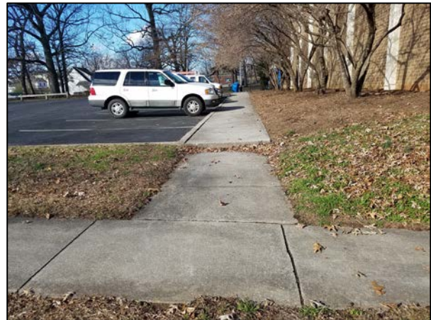
Step at Southeast Corner
