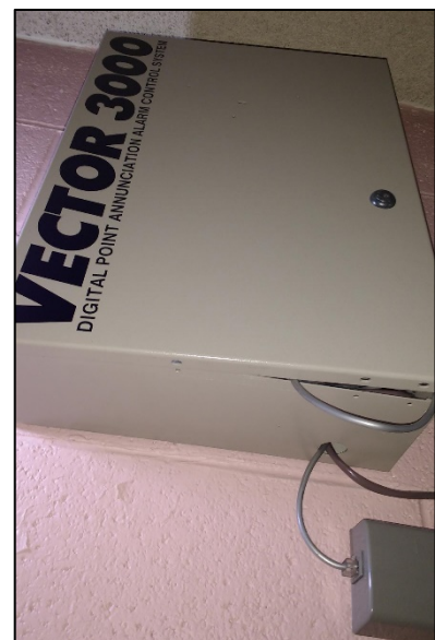
Fire Alarm Panel
