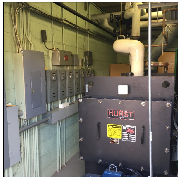
Subpanel and Breakers
