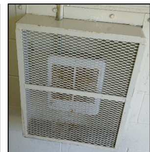
Toilet wall heater
