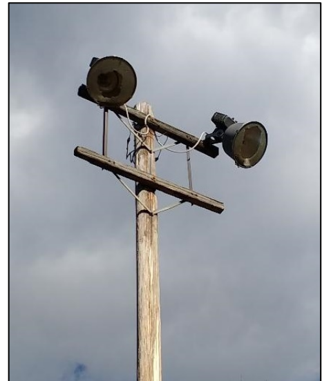
Damaged Ballfield Lights
