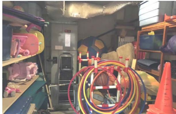
5-ton Air Handler
