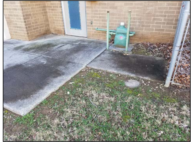
Gas and Water Service
