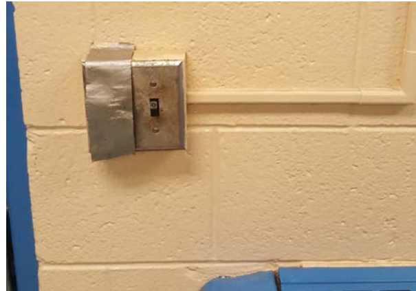
Typical Light Switch and Wiring
