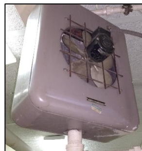
Toilet unit heater
