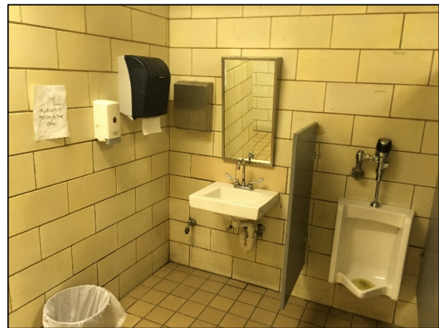
Typical Plumbing Fixtures
