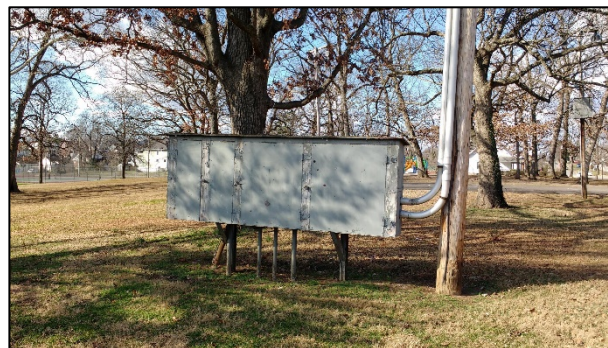
Ballfield Lighting Cabinet
