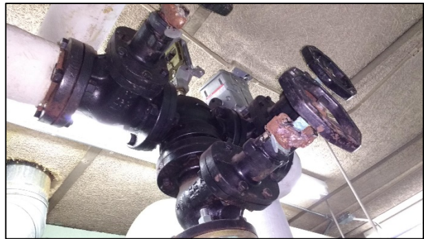
Boiler Mixing Valve
