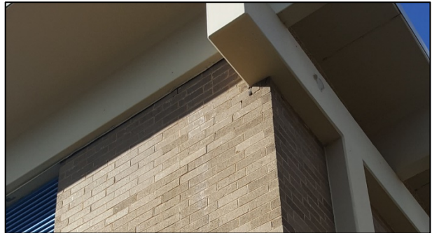
Location of Crack at Northeast Corner
