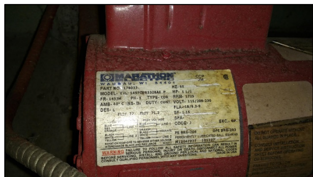
Heating Water Pump
