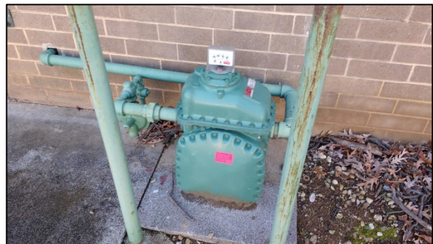
Natural Gas Meter
