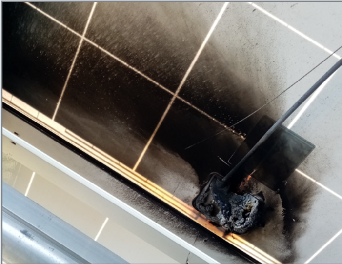
The image above shows a PV module at the project site with a junction box that melted due to electrical arcing.
