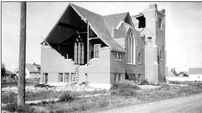
Three Forks church, following 6.6 magnitude Clarkston earthquake, June 1925. Photo by J.T. Pardee (courtesy USGS).
