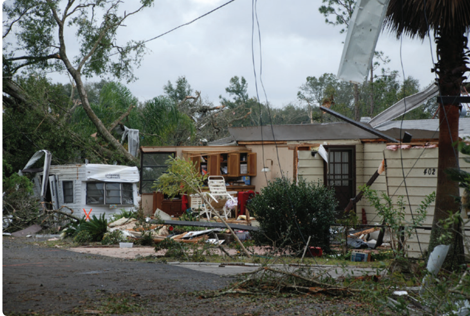
Fig. 27-13: Downed electrical wires are extremely dangerous and require that a safety area is established. Photo: courtesy of Captain Phil Kleinberg, EMT-P.
