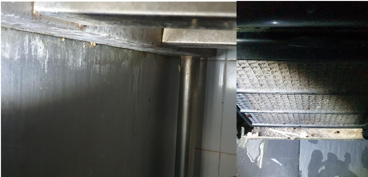
Cockroach infestation found underneath the hand washing sink (left) and chiller motor compartment (right) in the kitchen (Photos: SFA)
