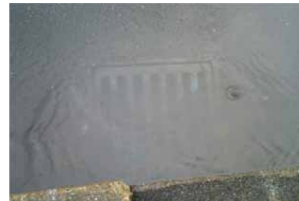
▲ Figure 2. Gullies frequently become overwhelmed, restricting any further water from entering the drainage system. (© Wilhelmina Drayton)
