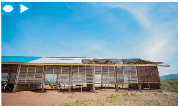
Lubile 1 Primary School in Tanganyika Province, Democratic Republic of the Congo, was destroyed when militia groups clashed and inhabitants deserted the village. Three classrooms made of tarpaulin are being installed with CERF support in February 2021 to allow students to resume classes quickly. UNICEF undertakes the construction of permanent classrooms. | 18 MAY 2021/UNICEF/JOSUÉ MULALA
