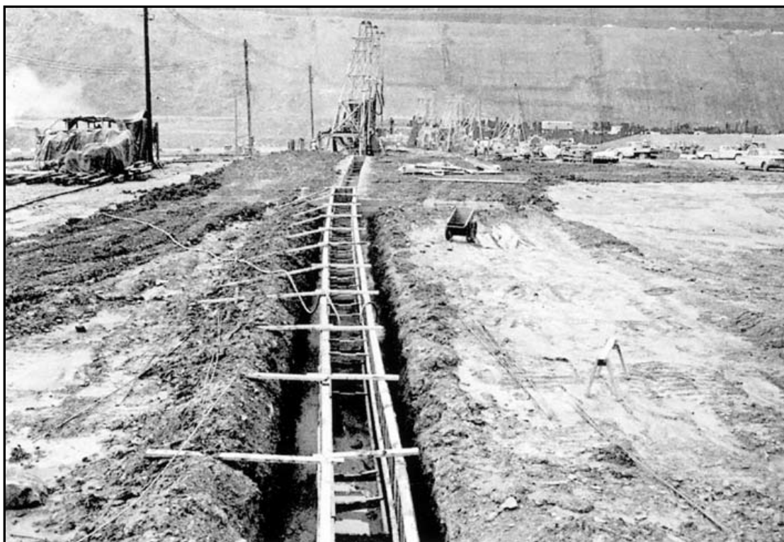
Figure 8-8: Seepage into the earthfill section of Kinzua Dam was prevented by constructing a trench three feet wide, 1100 feet long, and up to 160 feet deep on the upstream side. This was then filled with bentonite slurry to stabilize the side walls and then filled with concrete placed through pipes from the bottom up displacing the bentonite slurry. Source: Pittsburg District, U.S. Army Corps of Engineers.
