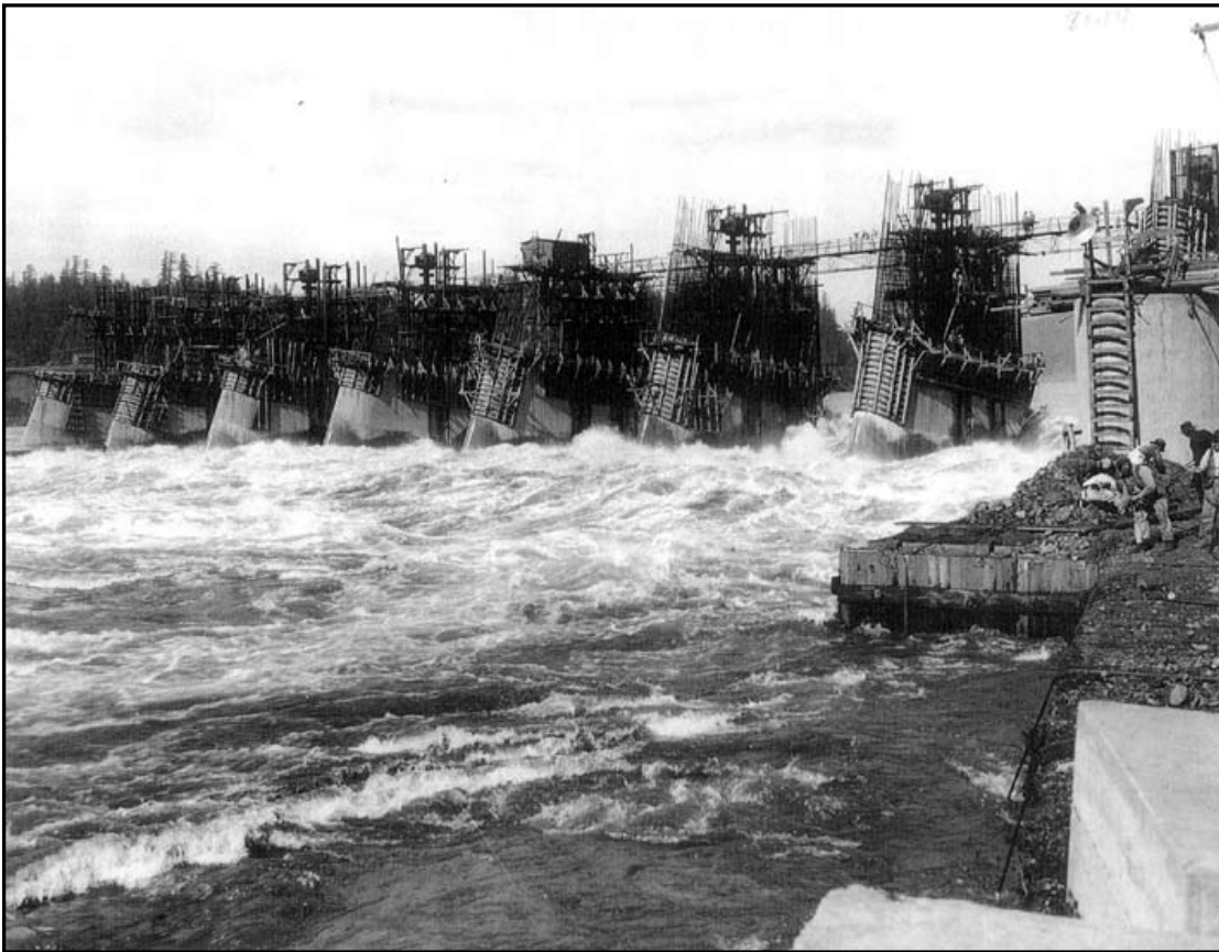
Figure 5-4: Turbulent flow between partially completed piers of Bonneville Dam during the flood season. Source: Records of the U.S. Army Corps of Engineers, Record Group 77, National Archives and Records Administration, College Park, Maryland.
