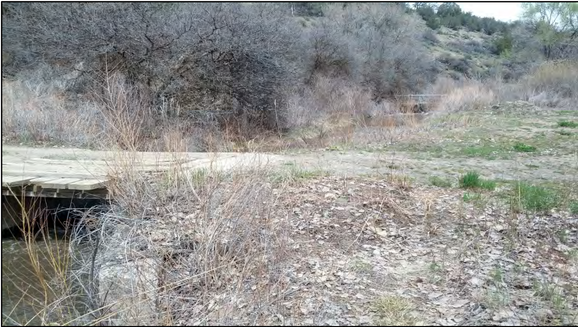
Photo 9. Bridge over existing canal; would be removed when the canal is piped. View northwest.
