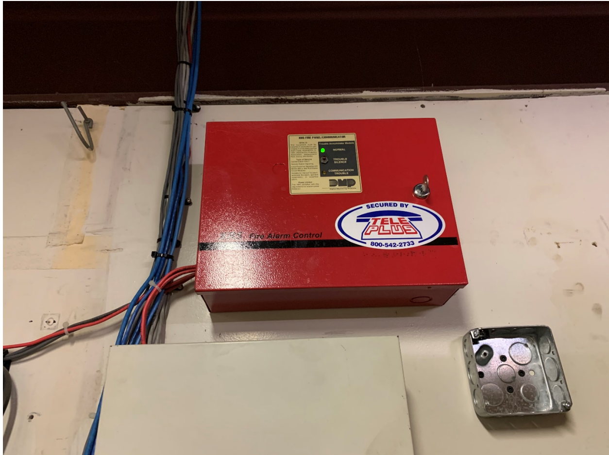
Hangar-21 Existing Fire Alarm Panel
