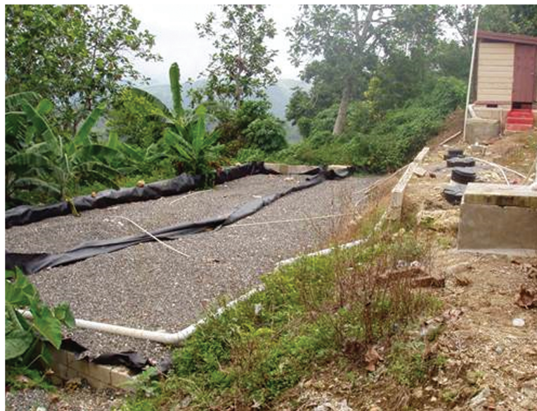
Figure 2. Two horizontal subsurface flow constructed wetlands (plants not yet planted) in parallel that treat septic tank effluent produced by a primary school in Jamaica (photo reproduced with permission from Edward Stewart (2005))
