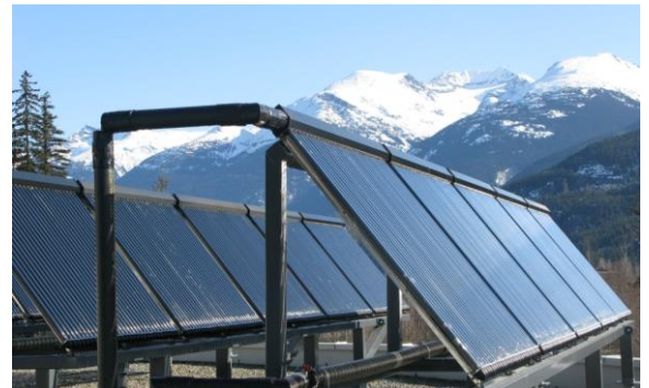
The solar thermal and geo-exchange installation at Meadow Park Sports Centre (2009) has reduced facility emissions by more than 400 tCO 2 e per year, catalyzed savings of $125,000 per year, and represents a major reason why the RMOW's corporate emission footprint is now 38% below 2008 levels.
